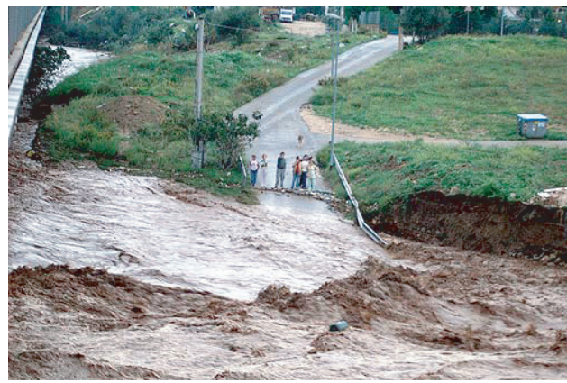
(h) Area of S. Rita di Bari. Road destroyed by flood.
