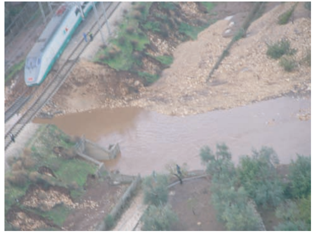
(b) Derailed Eurostar train. It is evident the undersized culvert.
