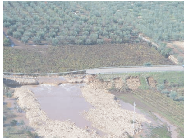
(j) Collapse of a road embankment between Cassano delle Murge and Bitetto.
