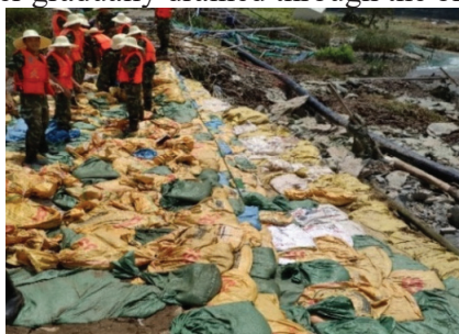
Figure 1. On-site photo of the breached seawall in Yacheng Town.
