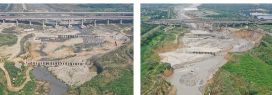
Figure 2. Failure of grade controls due to improper design
