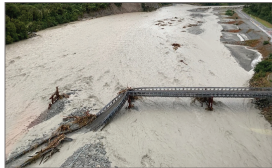
Figure 2. Waiho River bridge failure during the 2019 flood. The bridge suffered the combined influence of severe bed aggradation and local scour.
