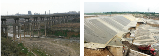
Figure 1. Damages and failures of instream structures caused by rapid bed degradation in mountain rivers.
