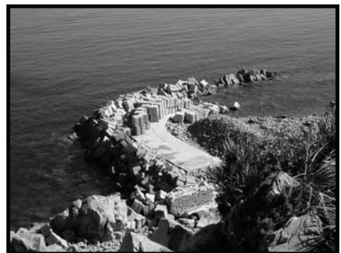
Figure 2: Destructed Breakwater during Construction
